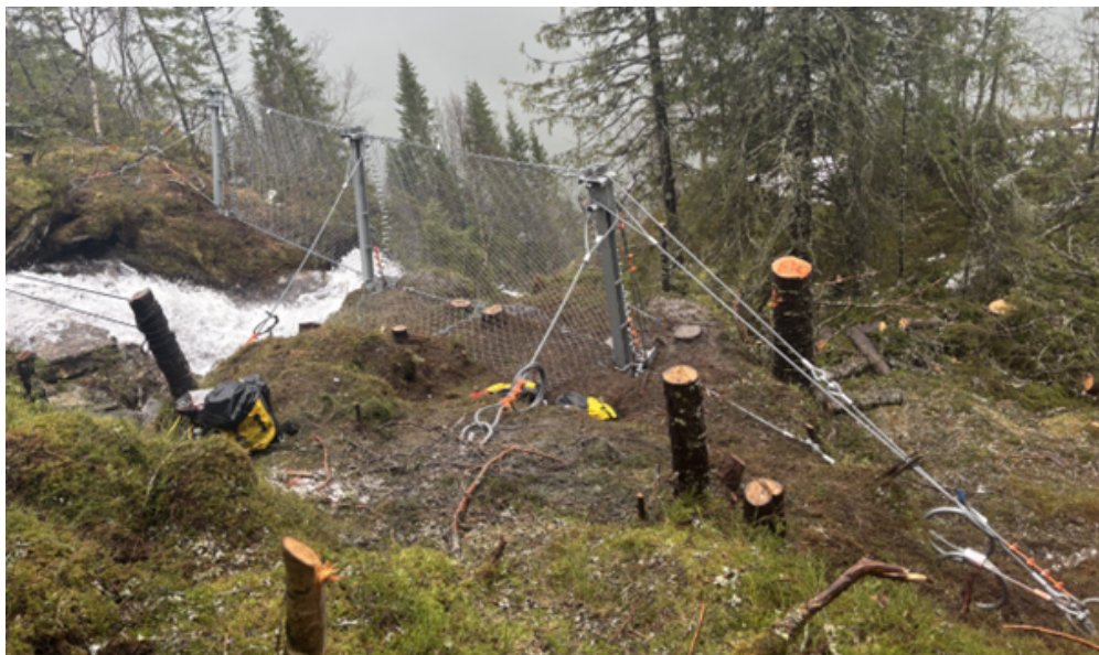
Figure 2 One of the flexible barriers installed along the railway line (Photo: Bane NOR).
