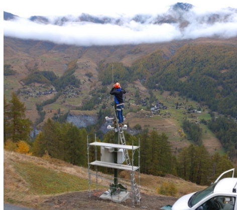
Figure 2 Installation of Doppler radar beside a mountain road in Evolène.
